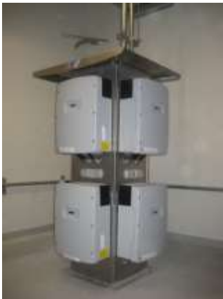
ST-42 Inverter Tree Used by Both Systems
