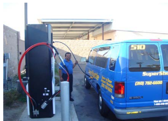
Upgraded Station in Operation
