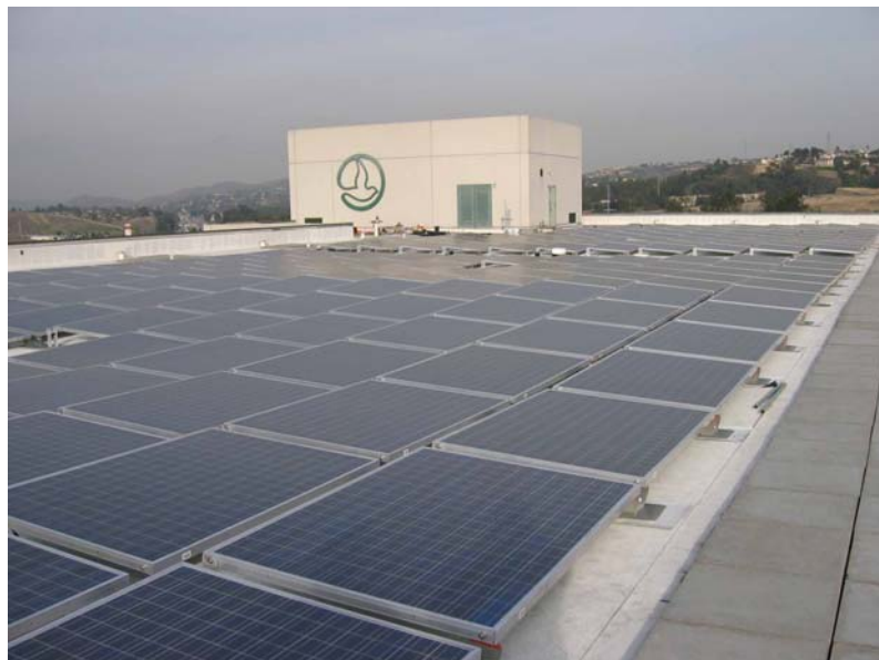
Figure 6: Solar Panels on SCAQMD Roof
