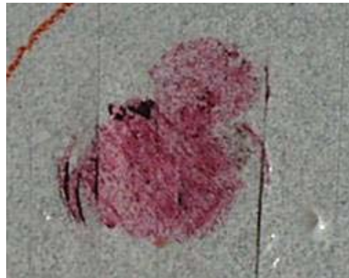
(Damaged) And White (Undamaged) Coating On Cylinder.
