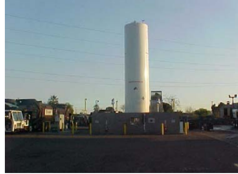
LNG Fuel Station and Storage Tank
