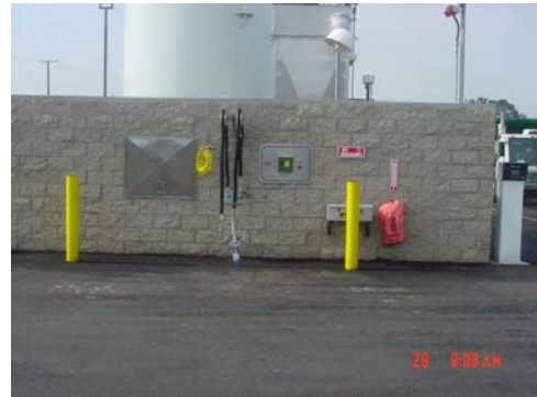
LNG Station Control Panel and Dispenser
