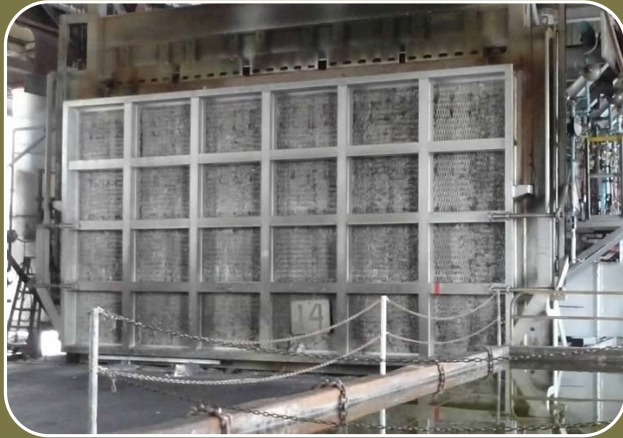
Furnaces Conducting Heat Treating
