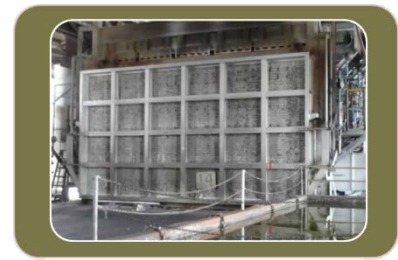
Furnaces Conducting Heat Treating
