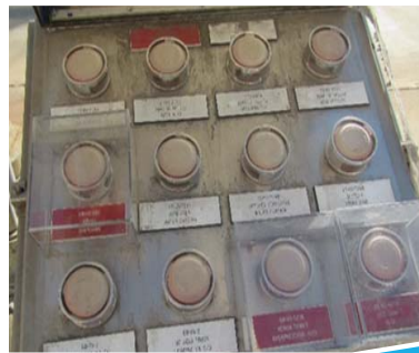
Emergency isolation block valve
