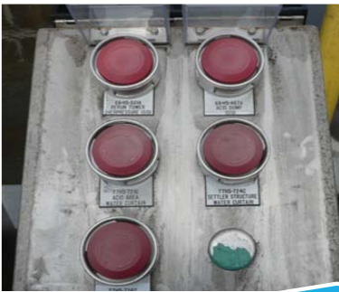
Acid evacuation system
