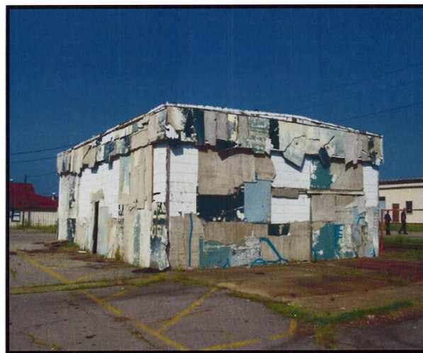
AACM2 building with added asbestos-containing Transite prior to demolition. (EPA photo)
