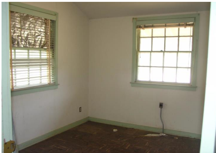
Interior of the AACM1 building shows the asbestos hazard (i.e., the asbestos-containing joint compound connecting the gypsum wallboard). 13 (EPA photo)
