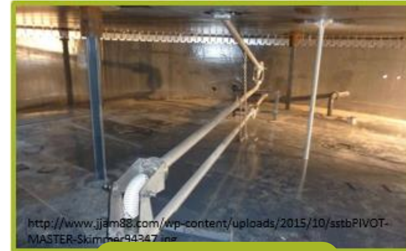
ROOF DRAIN Drains rainwater from roof
