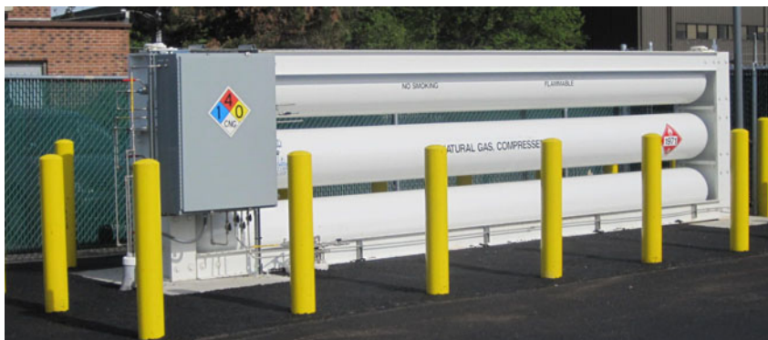
Figure 21 High Pressure Storage Tubes for CNG
