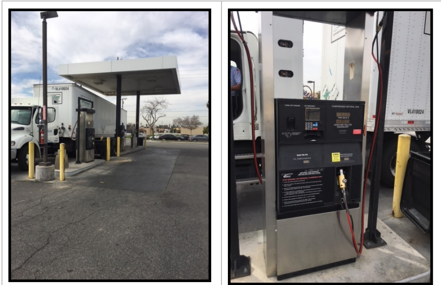
Figure 22 CNG Fueling Equipment Located on Pershing Ave., San Bernardino
