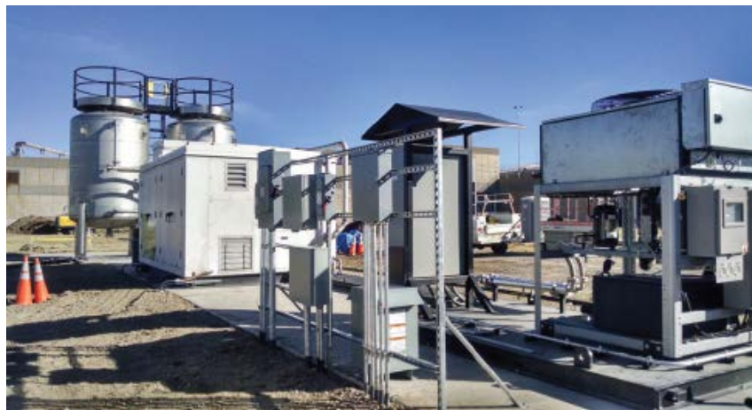
Figure D.2 Digester Gas Conditioning System in Grand Junction
