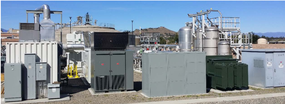
Figure D.1 Fuel Cell Installation at the Riverside RWQCP
