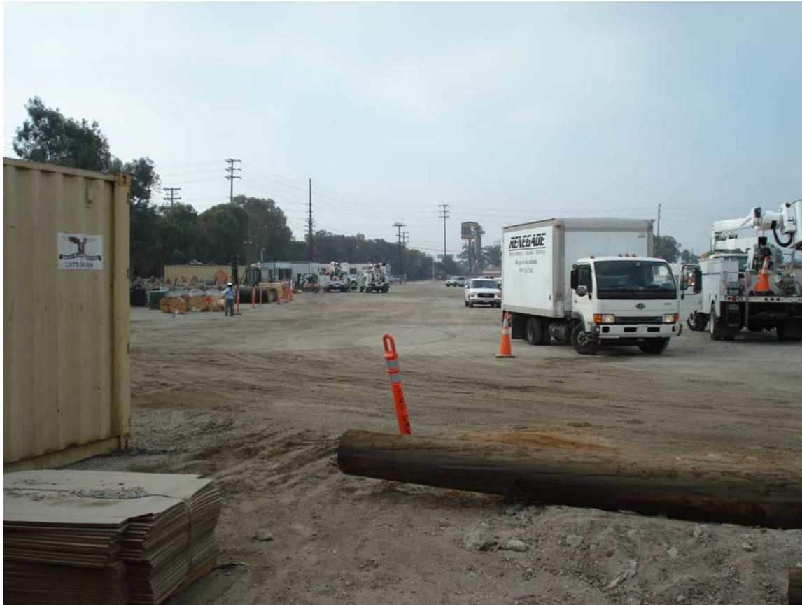
Figure 9: Looking south from northernmost edge of substation.
