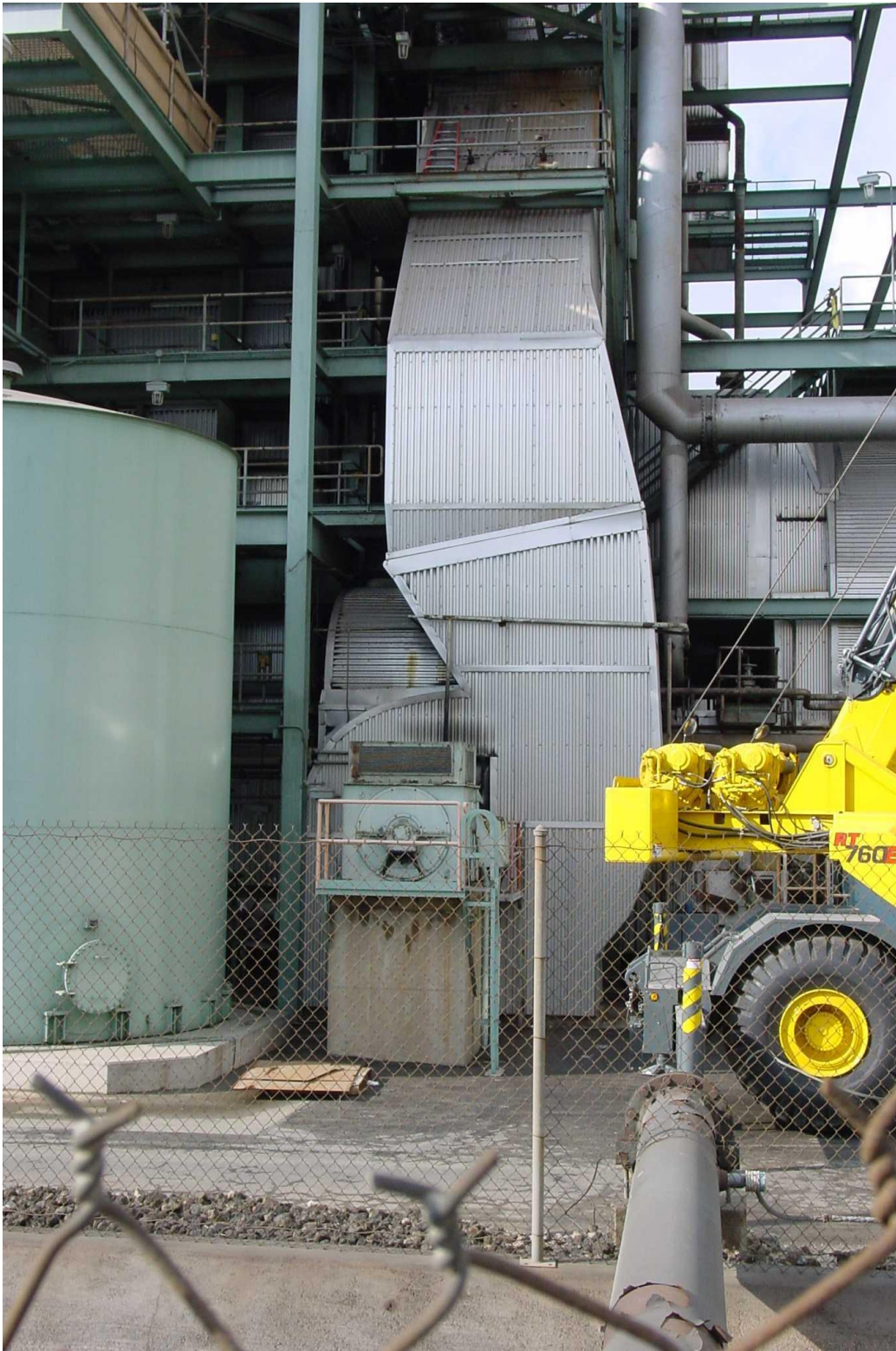
Ducting View and Location of Catalyst Installation
