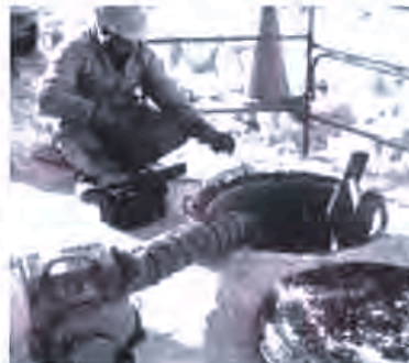
Continuous ventilation and testing are critical in any confined space with a harmful atmosphere.
