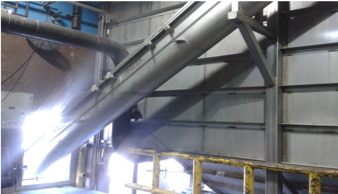
Typical conveyor system observed at a local rendering facility.
