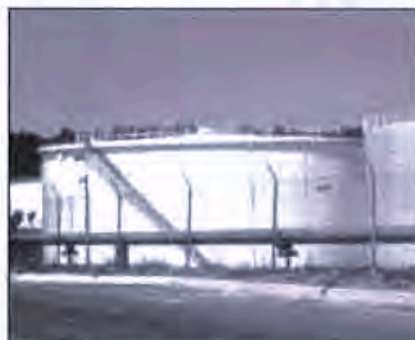
Chemical storage tank
