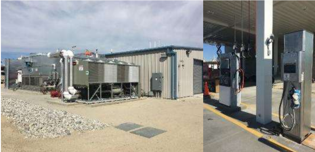
Figure 7: SunLine Transit Agency Onsite Hydrogen Fueling Infrastructure
