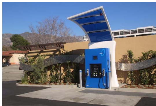
Photo of installed Hydrogen Station at La Canada Flintridge. Source: FirstElement Fuel, Inc.
