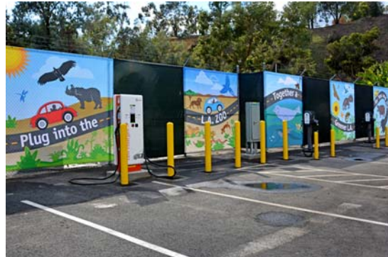
Figure 1: Los Angeles Zoo, DCFC and Level 2 EVSE
