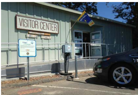
Figure 3: Leo Carrillo State Park Level 2 EVSE
