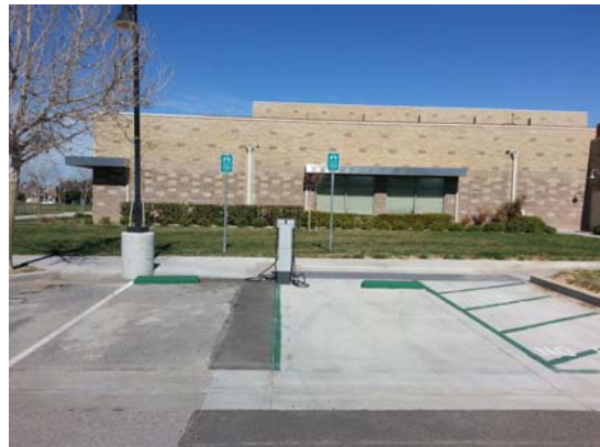
Figure 2: City of Palmdale Level 2 EVSE
