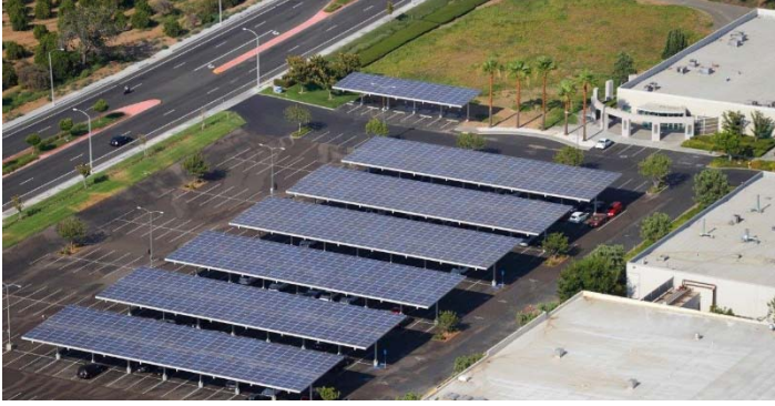
Figure 9: UCR's 4 MWs of Photovoltaic Panels Constructed for Sustainable Integrated Grid Initiative
