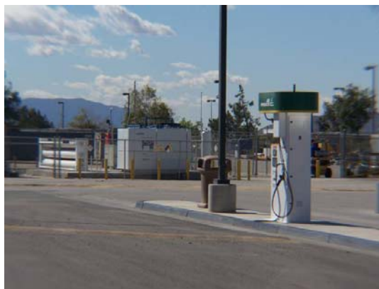
Figure 2: Riverside Electrolyzer Station
