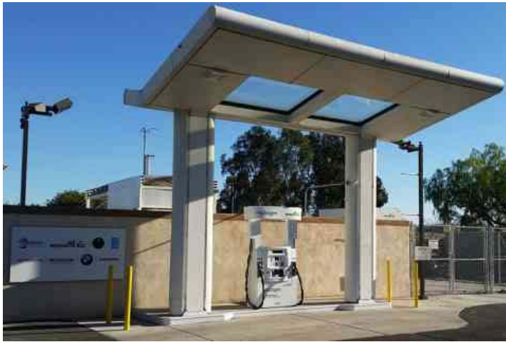
Figure 16: Existing Dispenser Installed November 2015
