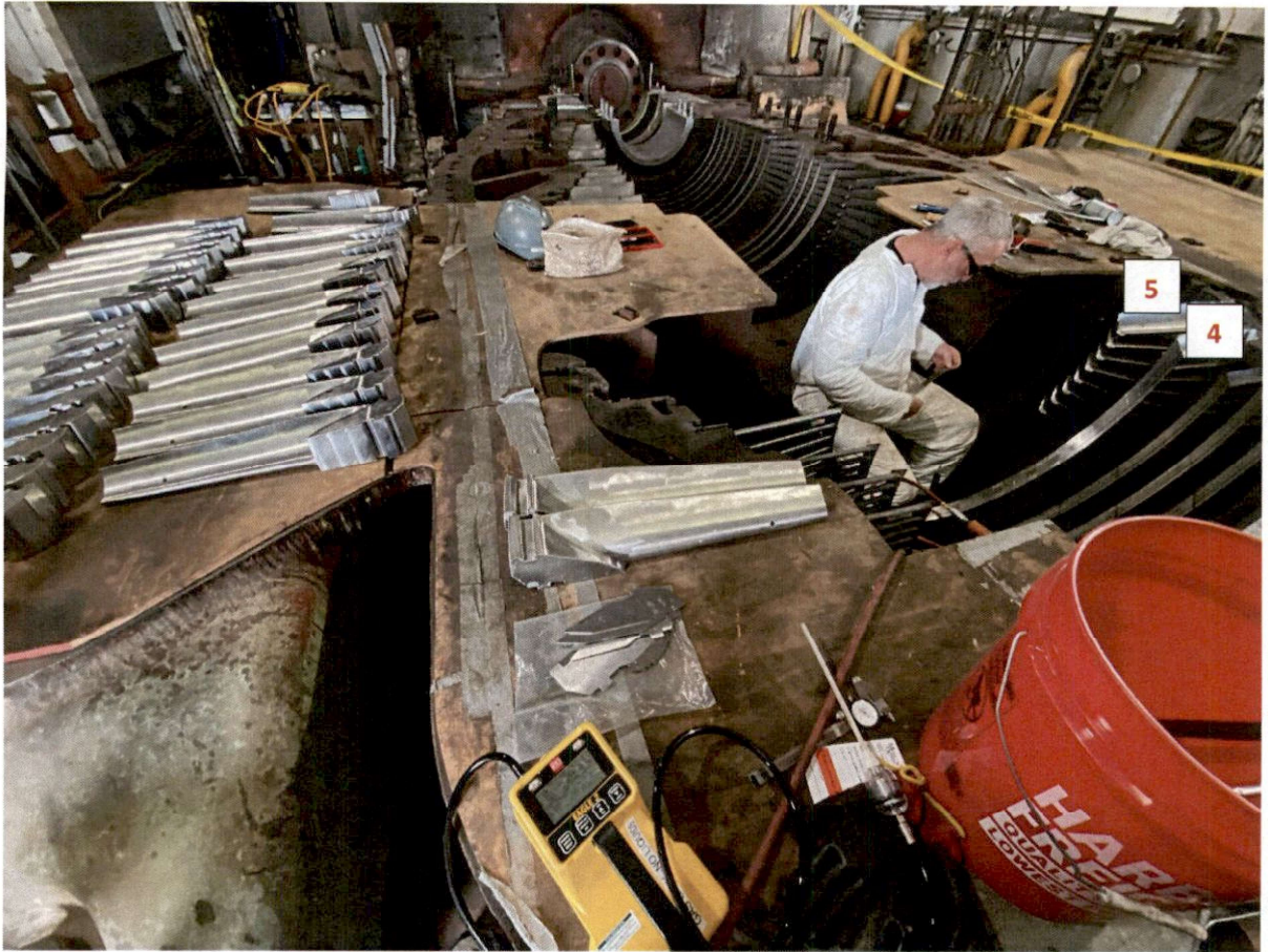
June 17 th , 2023 – GE Installing new Stage 4 and Stage 5 Stationary Blades on Lower Case , Generator End
