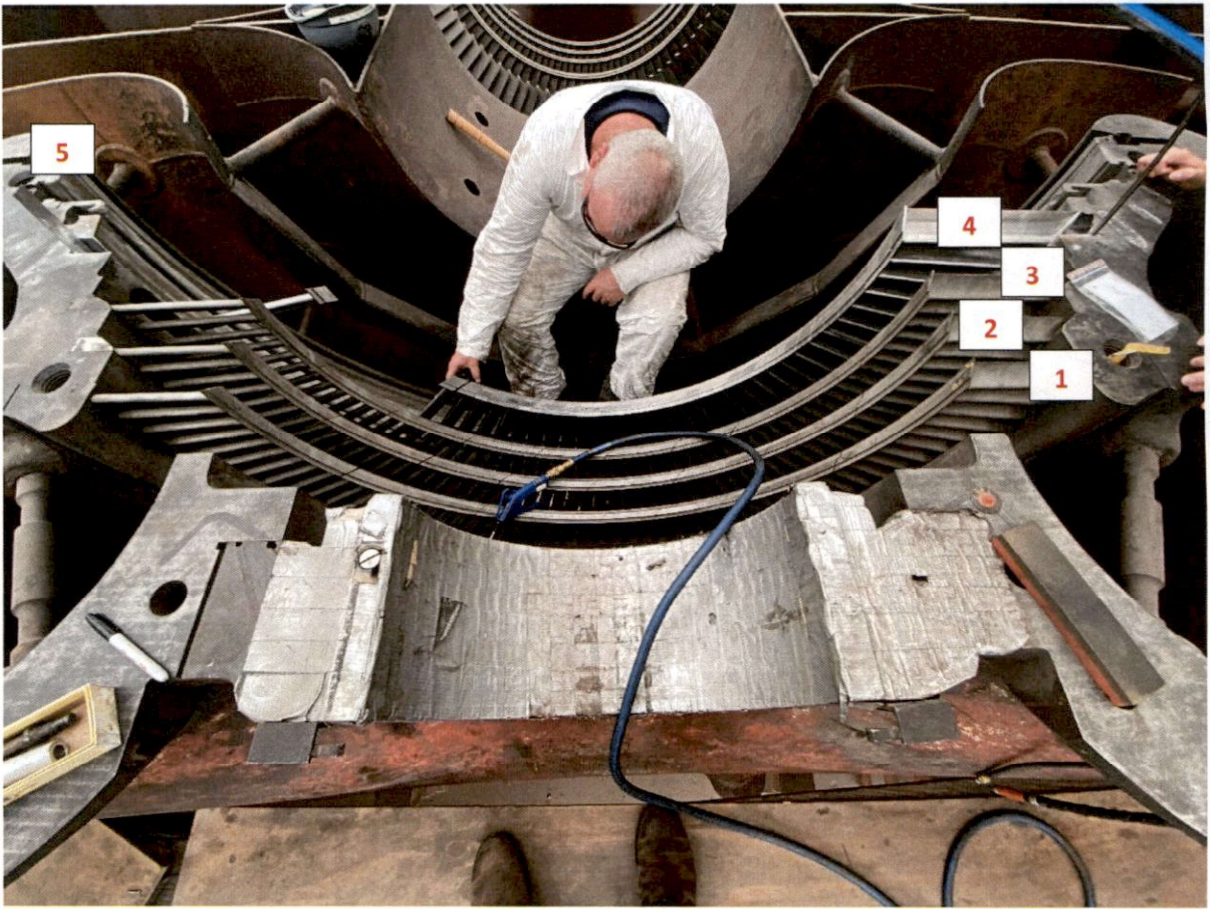
May 25 th , 2023 – GE installing new Stage 4 Stationary Blades on Top Case, Generator End
