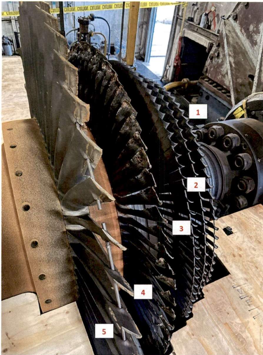
December 29, 2022 – Damaged Rotating Stage 4 & 5 Blades on LP, Generator End
