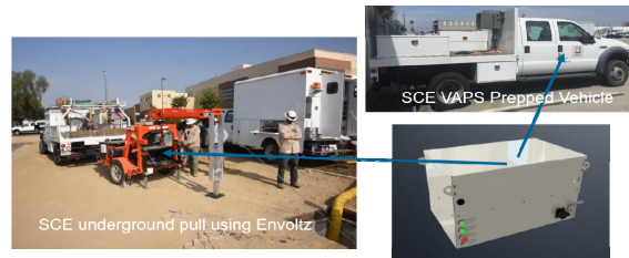
Figure 1. VAP System by Envoltz, LLC
