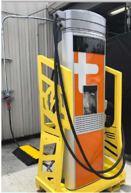
Figure 13: ChargePoint CPE 250 Skid-Mounted Mobile Charger with Protective Cage
