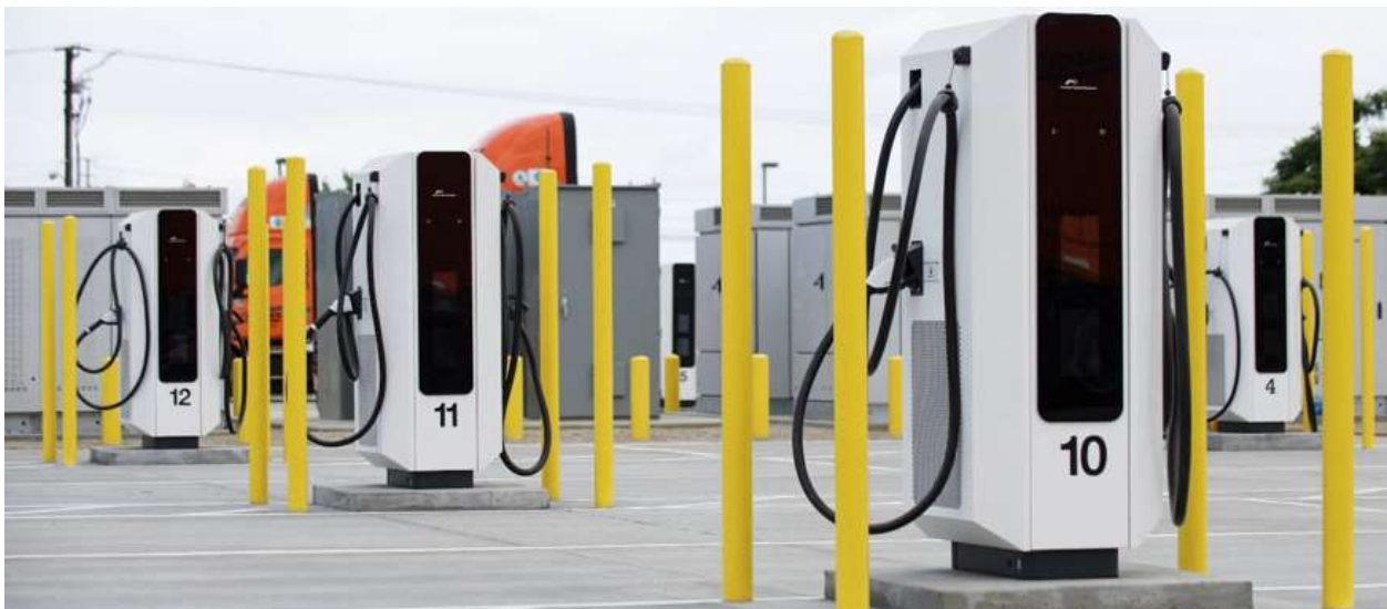
Figure 8: Schneider Deployed Sixteen 350 kW DC Fast Chargers Manufactured by Power Electronics
